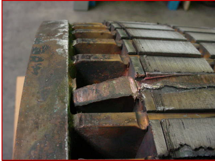
Fig. 9.5: Defect rotorstaaf-kortsluitring verbinding.
